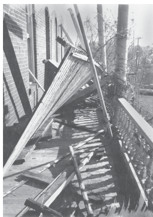
Twisted balcony railings attest to the strength of the winds.
