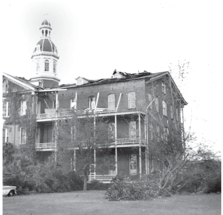
Downed trees and damage to roof and balcony on west wing of the Academy.
